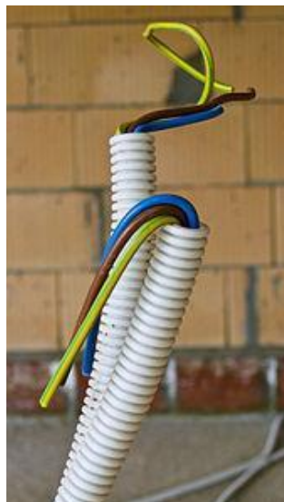
Colored wires in a flexible plastic electrical conduit commonly found in modern European homes
