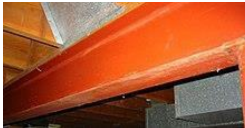
A metal I-beam used in this case to support wooden beams in the house.
