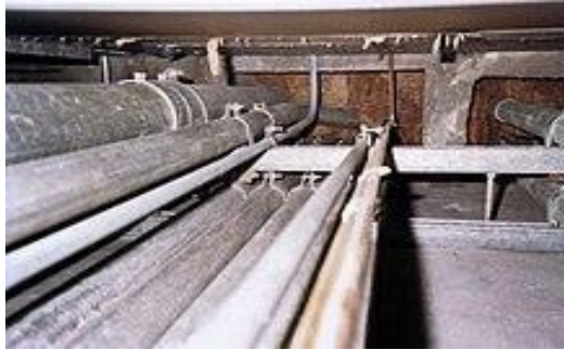
Electrical conduit risers seen inside the fire rated shaft
